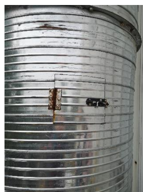
排气筒出口监测孔
